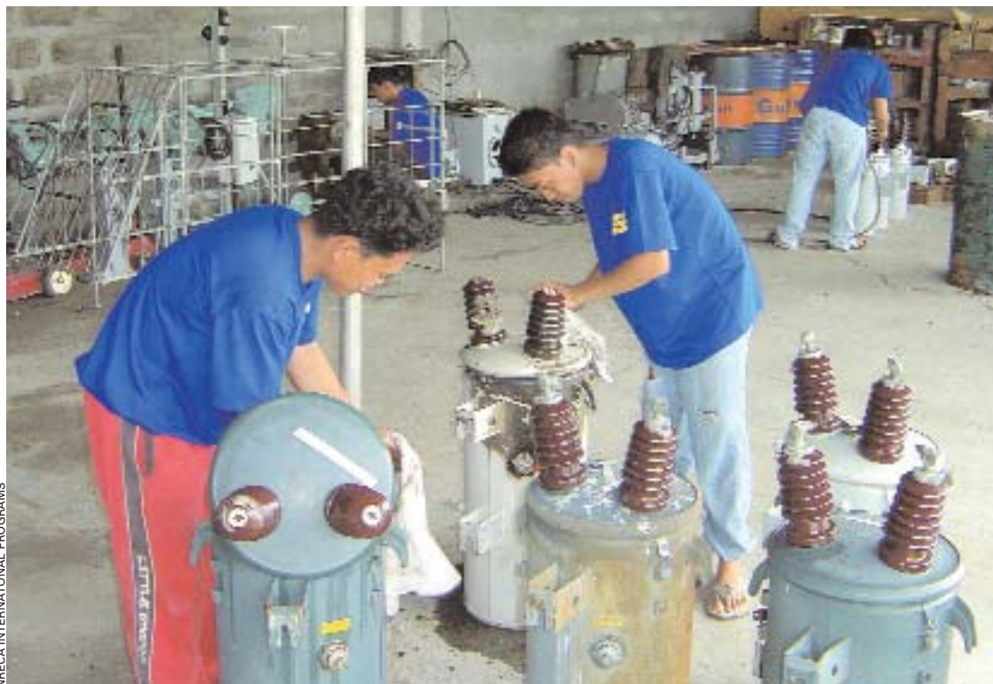
Employees at Davao Del Sur Electric Cooperative in the Philippines refurbish donated transformers, thanks to a helping hand from Big Rivers Electric Corporation, a Kentucky generation and transmission co-op.
